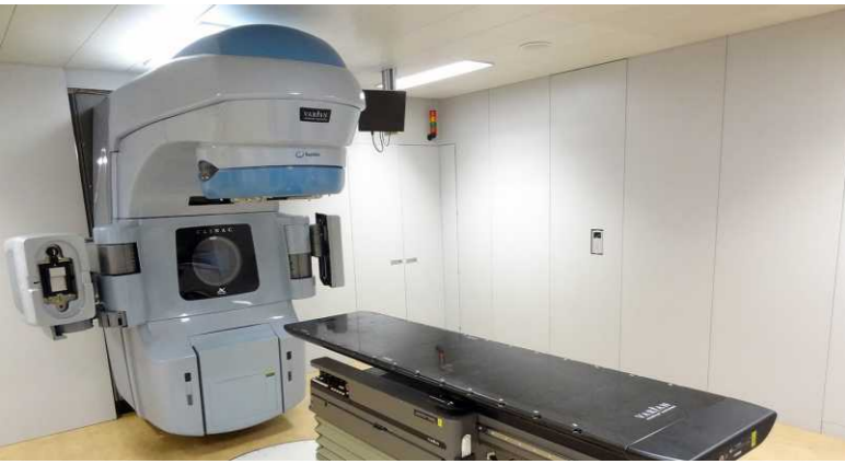
Linac Machine in a radio - active bunker
