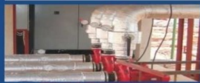
PRIMARY PUMP INSTALLATION AT NIGERIA JUDICIAL COUNCIL
