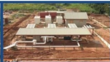
HEAVY DUTY HVAC INSTALLATION AT THE NIGERIA JUDICIAL COUNCIL HQ, IN ABUJA
